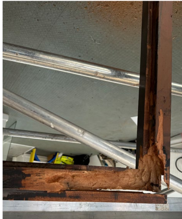
Window removed from frame and rot discovered
